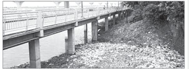
Garbage dumped at Anta Ghat.
