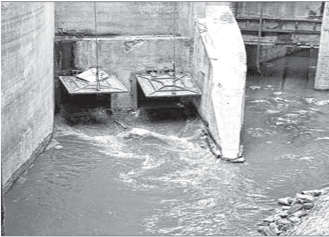
The sewage treatment plant at Anta Ghat
